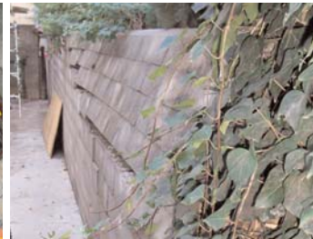
Side Wall Damage
