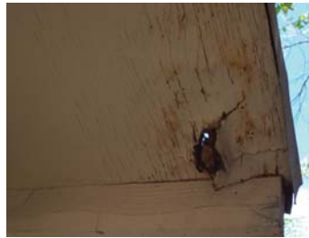
Roof Damage from Rain
