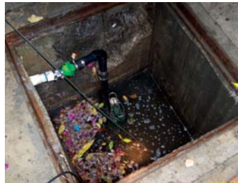
Broken Sump Pump
